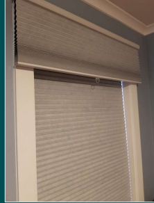
Honeycomb blinds installed inside the window frame
